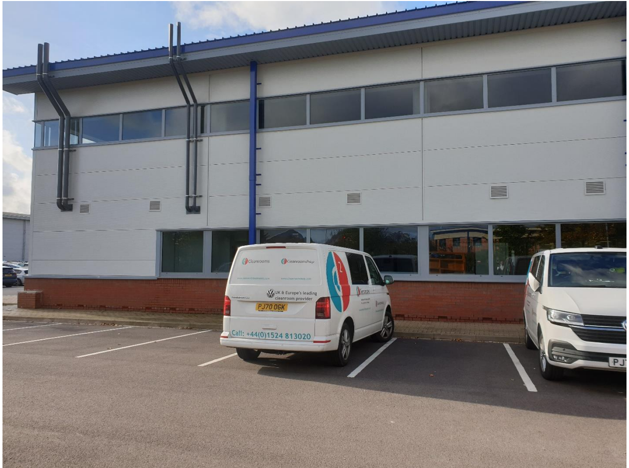
Figure 3 – The new flues on the north east side of the Orbis building
